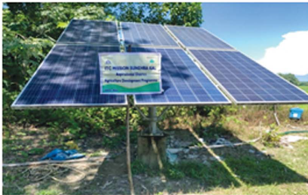
Fig: Solar energy installation for irrigation
