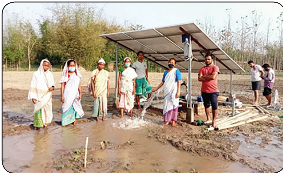
Fig : Solar Pump installed at Manipur village, Morigaon
